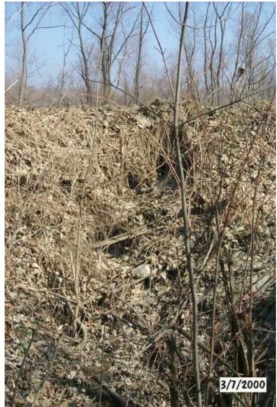
Erosion around culvert, Farr Road.
