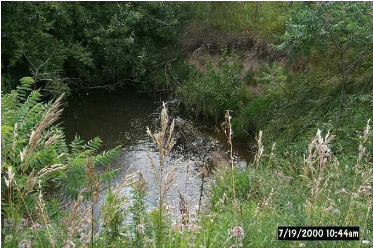
Blowout downstream of culvert.
