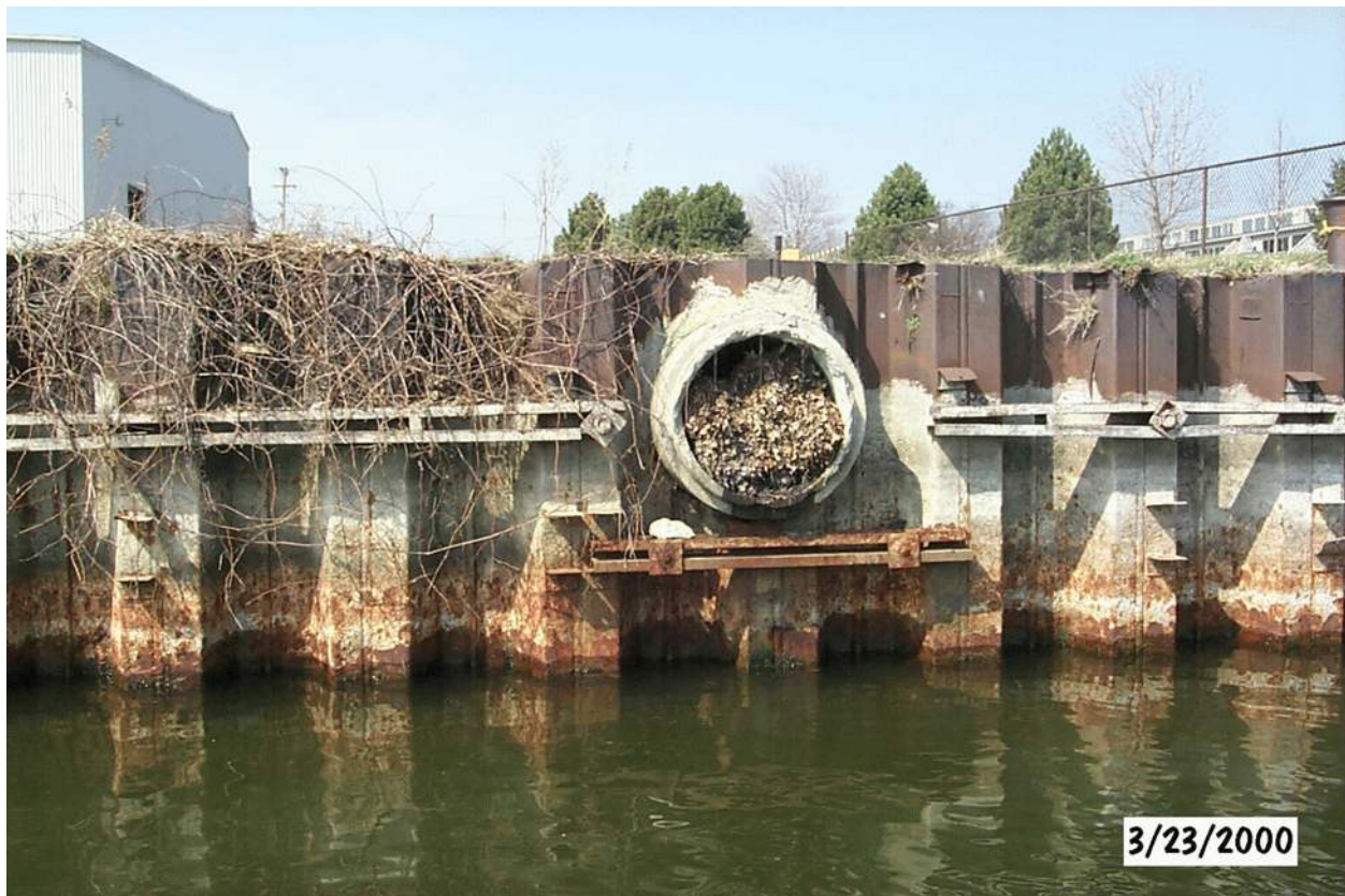
Figure 22. Storm sewer outlet to Spring Lake.
