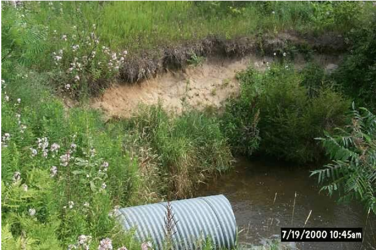
Blowout downstream of culvert.
